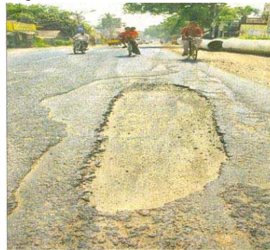
Conventional Bitumen Road at Madurai, Tamil Nadu Battered By Heavy Rain
